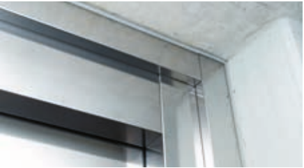
Panel between door frame and wall
